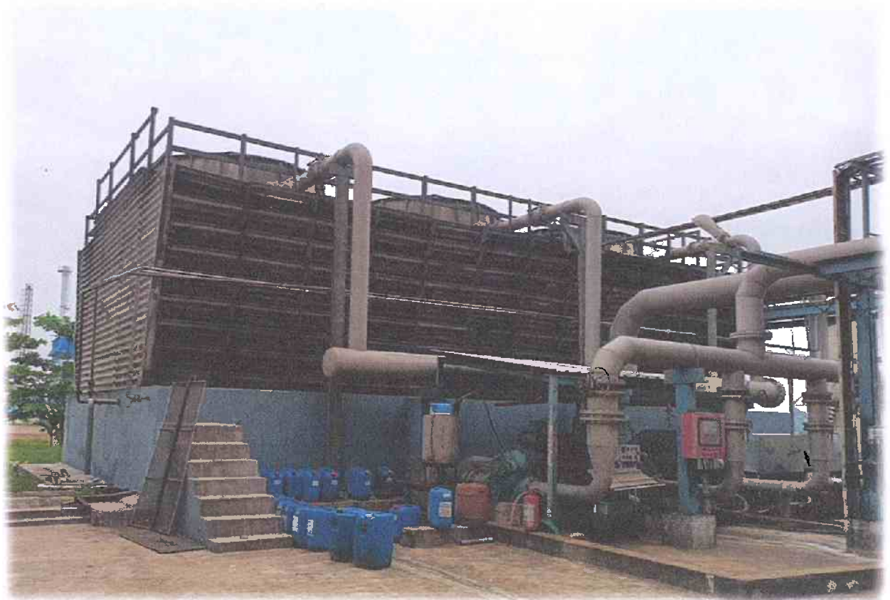
Annexure-I: Pictures of ETP & Cooling Tower
